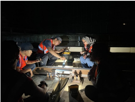
Hands on training... Sarawak Metro's young engineers and apprentices performing maintenance works at MRT Kuchai
