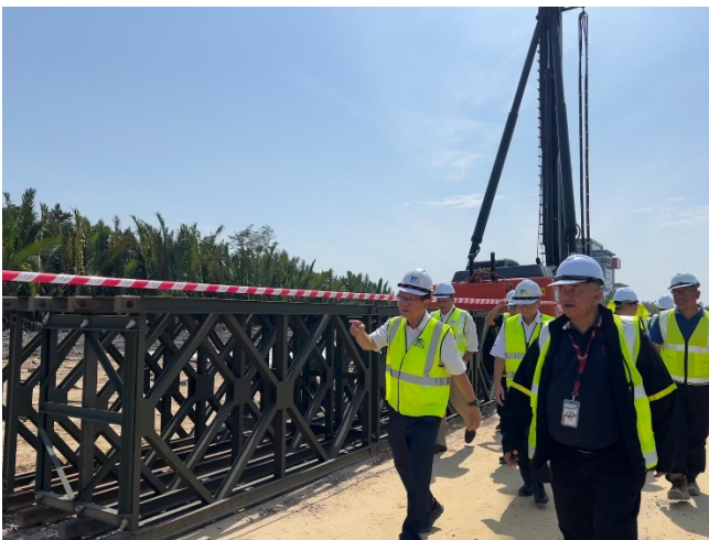
Minister for Transport Sarawak, Dato Sri Lee Kim Shin (left) inspects the progress of the Sg Kuap bridge.
