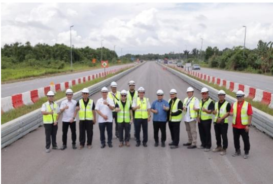
File photo of Minister for Transport Sarawak Dato Sri Lee Kim Shin (6 th right) and officials from Ministry of Transport Sarawak and Sarawak Metro during a visit to the Blue Line ART guideway construction site in Kota Samarahan
