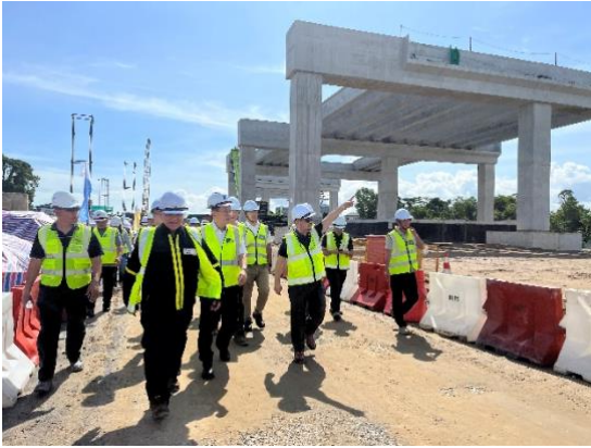
File photo of Mazli (3 rd right) with Minister for Transport Sarawak Dato Sri Lee Kim Shin during a visit to the construction site of the ART Interchange Station at Simpang Tiga
