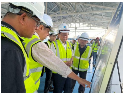
Lee Kim Shin (2 nd from right) being briefed on the construction progress of Simpang Tiga Interchange Station, while Mazli (right) looks on.
